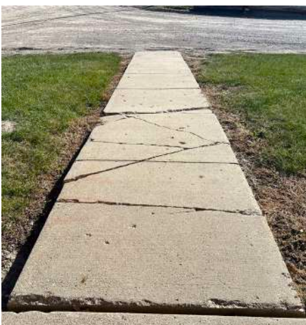
Deteriorating concrete sidewalk
