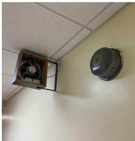
Bell and PA devices - may be non-functioning and/or abandoned
