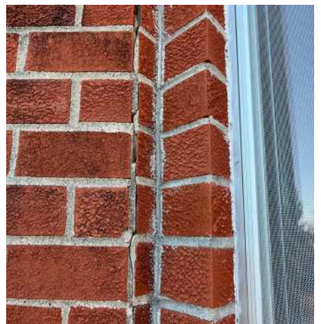
Failed mortar on 1982 facade
