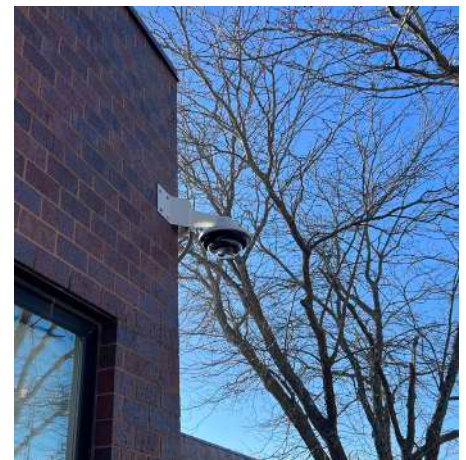
Exterior Surveillance Camera
