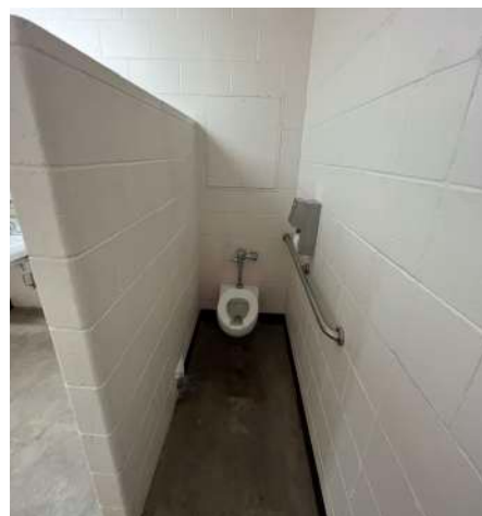
Non-ADA stall at Jr/Sr High locker room
