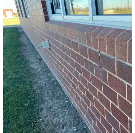
Brick facade; possible moisture intrusion below windows
