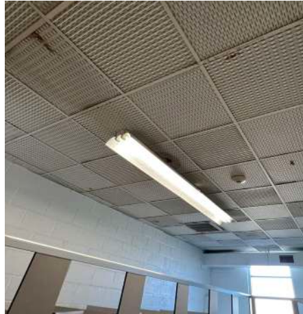
Surface-mounted fluorescent light fixture (1958 restroom)
