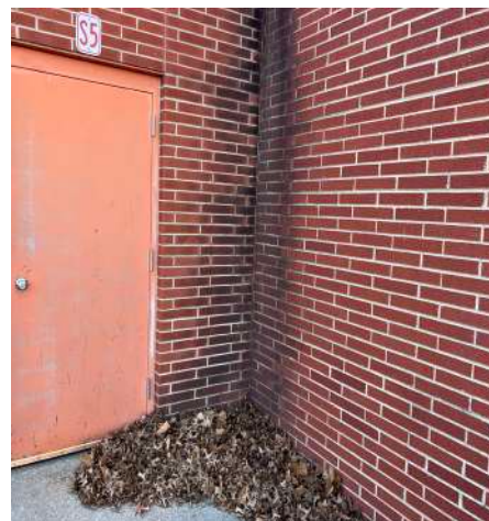
Staining and moisture concern where '88 and '58 bldgs meet
