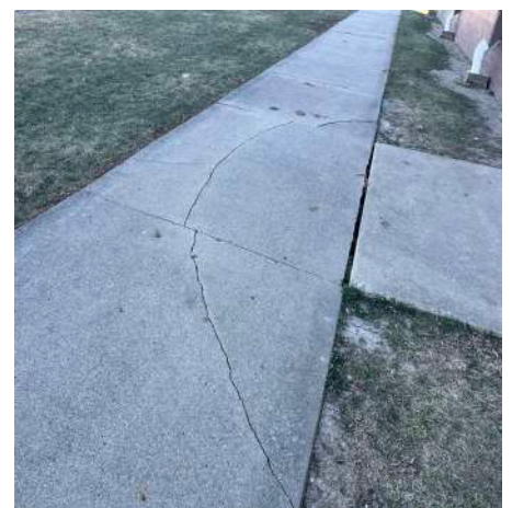
Concrete sidewalk is sloped towards building creating drainage issues
