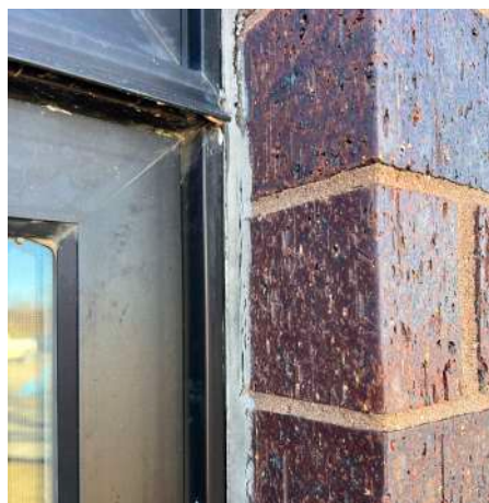
Window caulking in fair to poor condition
