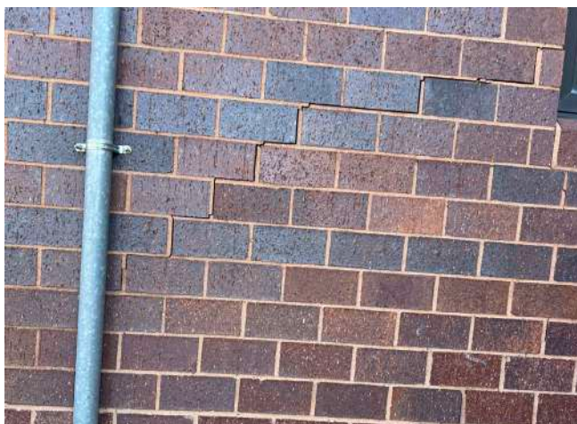
Contiguous crack along mortar line of exterior brickwork outside room 1111 (staff lounge/workroom)
