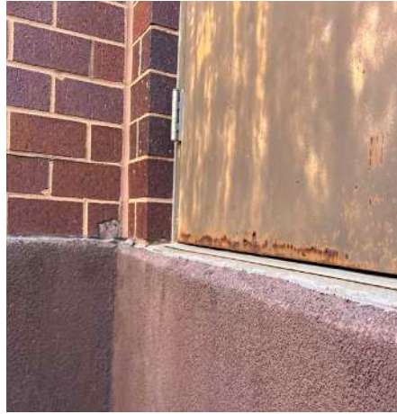
Rusting metal service door
