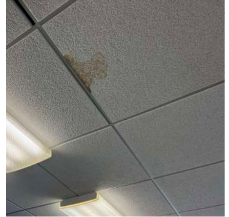
Stained ceiling tile (ceiling from 2007 renovation)
