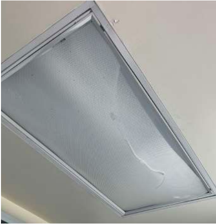
Recessed fluorescent Light Fixture (cracked diffuser lens)
