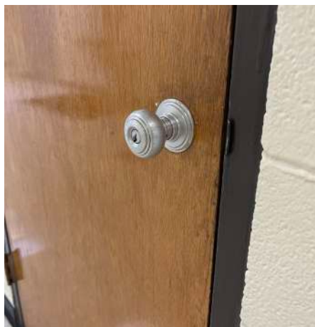
Non-ADA compliant knob-style door hardware
