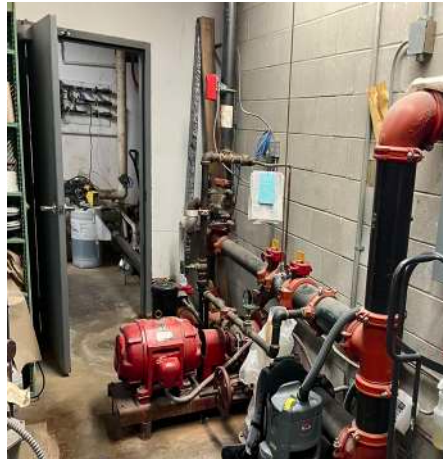
Jr/Sr High Fire Pump
