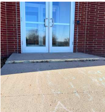
Settled sidewalk causing lip/trip hazard at concrete door stoop
