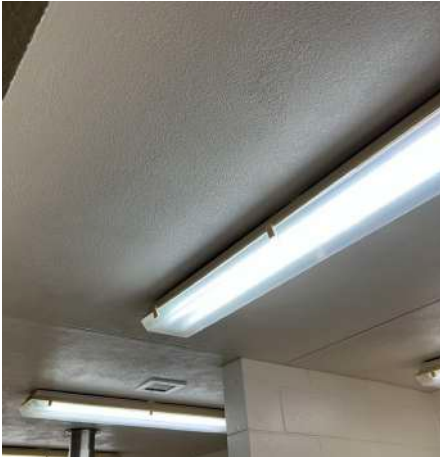
Surface Mounted Fluorescent Light Fixtures
