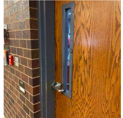
Metal door fram showing wear patterns around door handle
