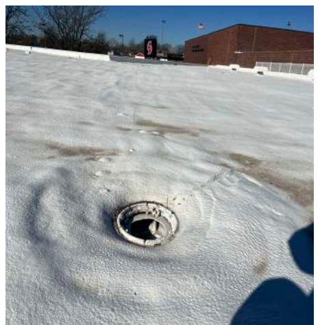
Recently spray-foamed roof; missing roof drain dome
