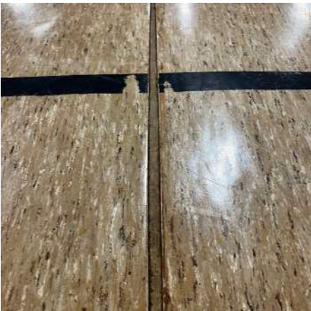
Rolled vinyl floor in gym separating at seams (asbestos containing)
