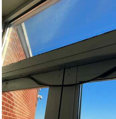
Loose weatherstripping on exterior door
