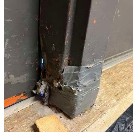
Rusted center mullion at exterior door in gym breezeway
