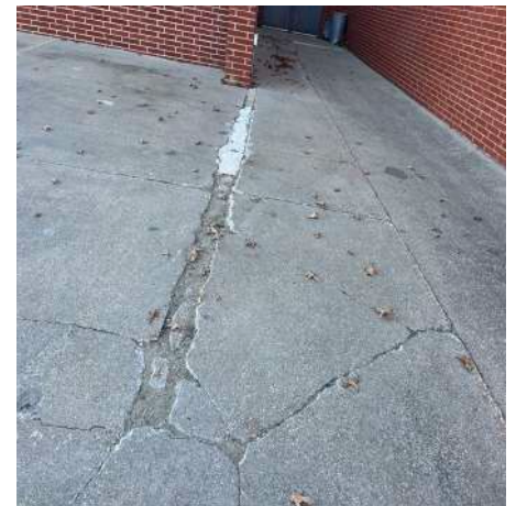
Major cracking at west parking lot
