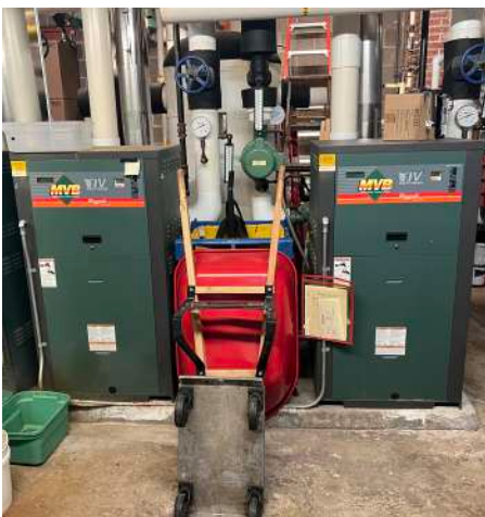
Steel Water Tube Boilers (2013)
