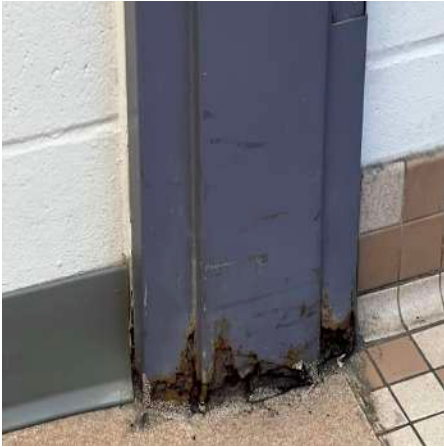
Rusting door fram at restroom entrance near commons
