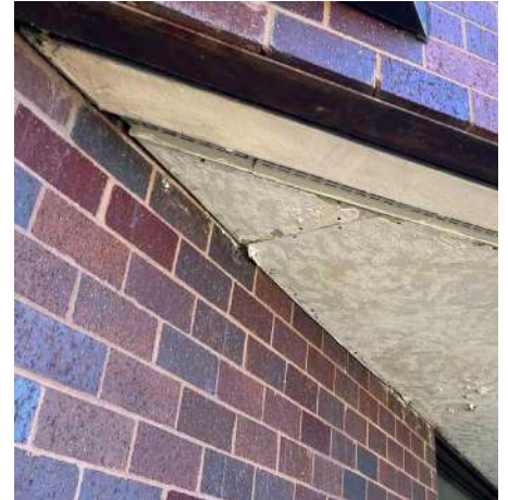
Flaking paint at main entry soffit (moisture concern)
