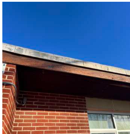
Peeling paint on wooden fascia (1957 addition)
