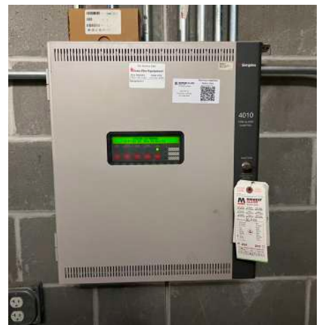
2003 North Elementary Fire Alarm room
