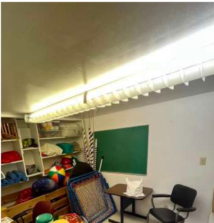
Louvered fluorescent light fixture
