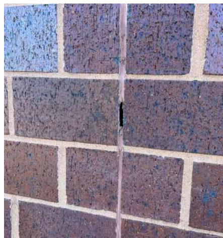
Hole in caulking in expansion joint
