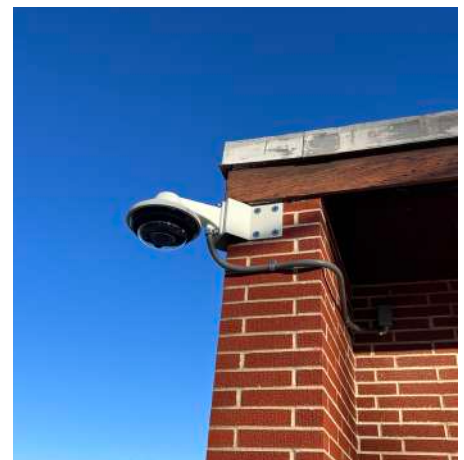
Exterior Surveillance Camera
