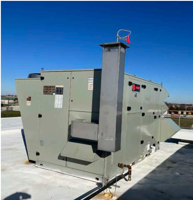
New Aux. Gym Rooftop Unit (2023)
