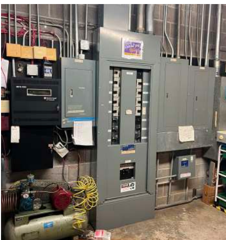
Main Electrical Switchgear
