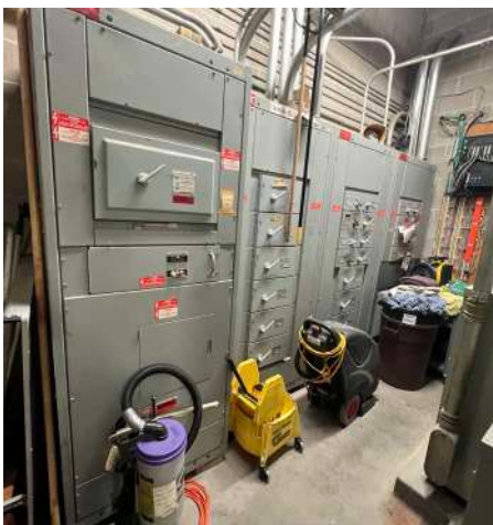
1986 Main Electrical Switchgear
