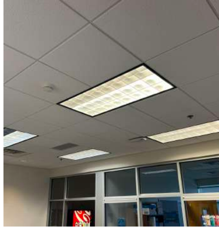
2x4 Fluorescent Parabolic Troffer Light Fixtures
