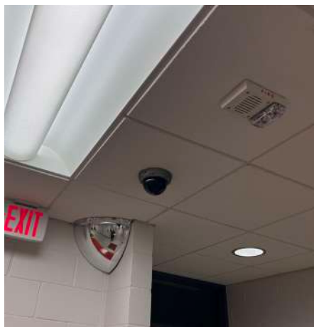
Interior Surveillance Camera
