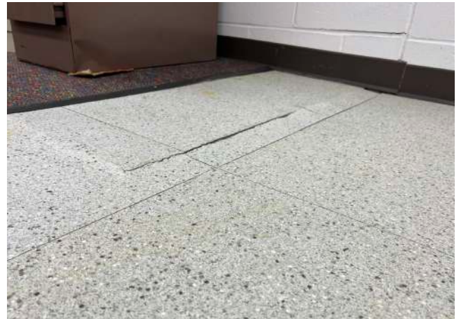
Floor settling in room 1123
