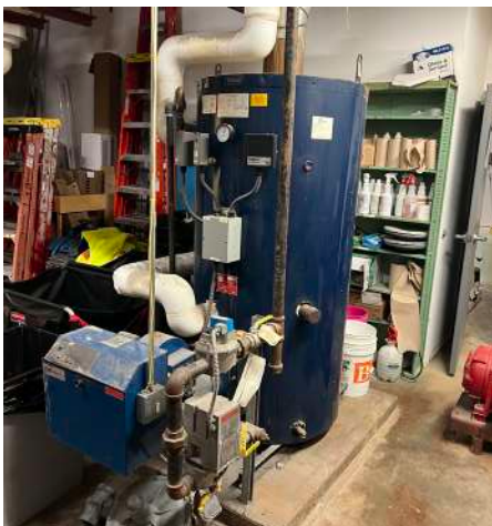
Jr/Sr High Boiler
