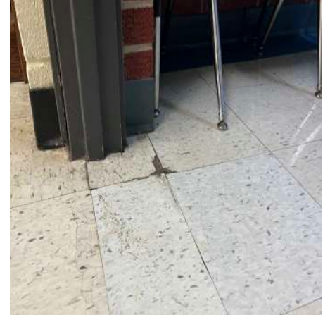
Cracked/chipping VCT floor
