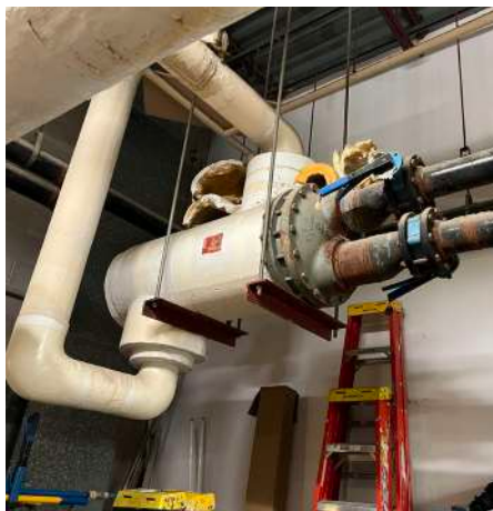
Heat Exchanger (original to construction)
