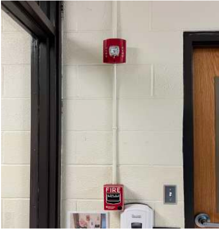
Fire alarm pull station with horn/strobe
