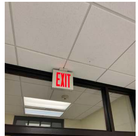
Corridor Exit Signage
