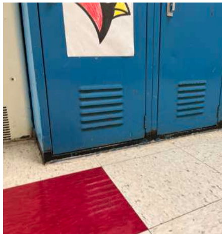
Lockers in hall rusting at base
