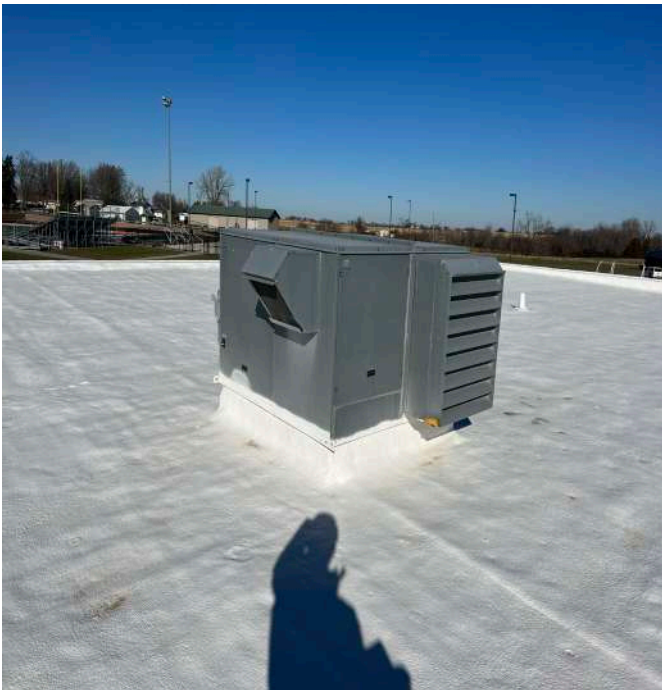
Energy Recovery Ventilator (ERV-2)
