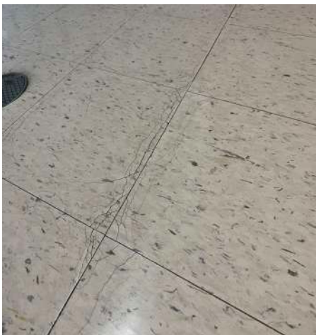
Cracked VCT floor
