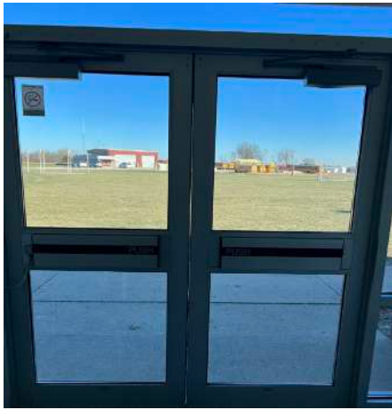
Daylight visible through door gap; missing weatherstripping
