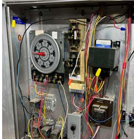
HVAC Control Panel
