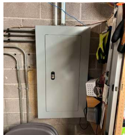
Newer Electrical Subpanel (2003)
