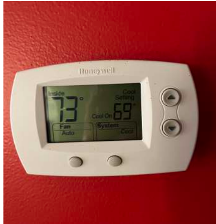
Honeywell Standalone Electric Thermostat
