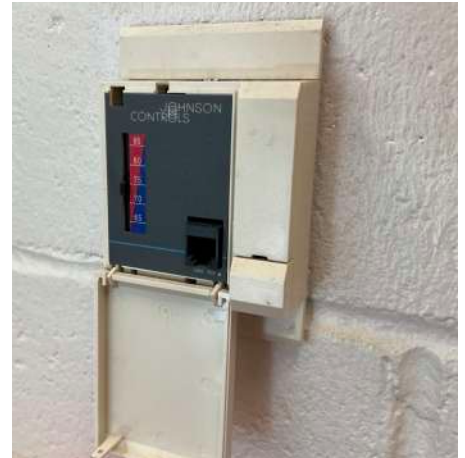
Johnson Controls DDC Thermostat
