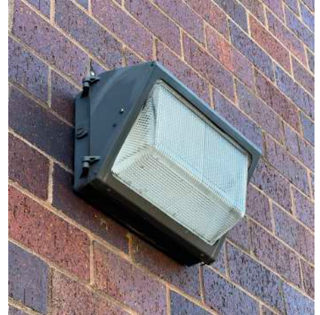
Exterior Metal Halide Lighting
