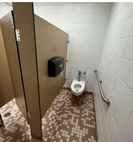
Non-ADA stall at Jr/Sr High restroom
