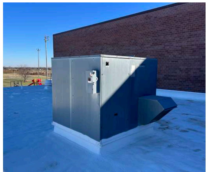
Energy Recovery Ventilator (ERV-1)
