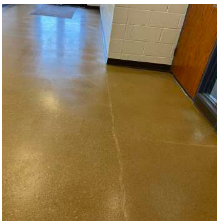
Epoxy Flooring in Halls
