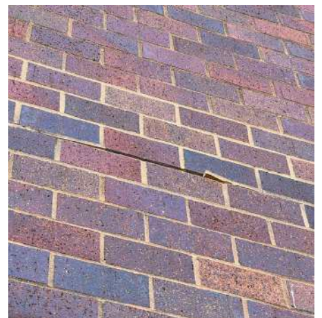
Missing/damaged mortar on south-west wall of main gym
