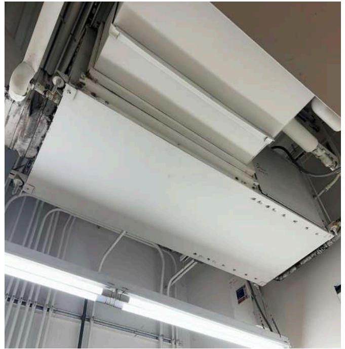
North Elementary Heat Pump
