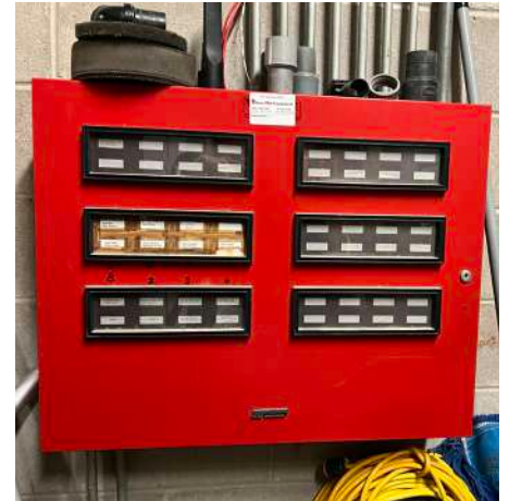
Abandoned Jr/Sr High Fire Alarm Panel
