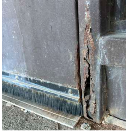
Rusting door fram at main entry vestibule
