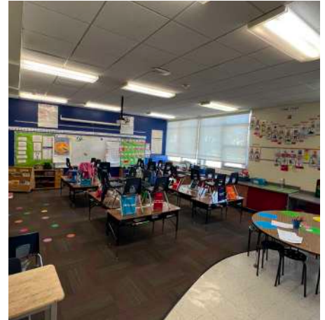
4 foot surface-mounted wrap-around fluorescent light fixtures
