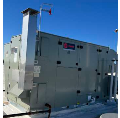
Main Gym Rooftop Unit (2023)
