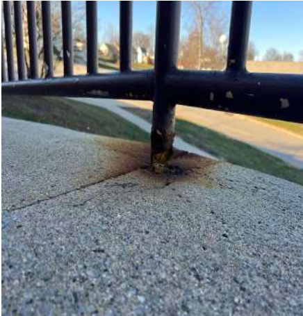
Rusting railing post at 2003 addition
